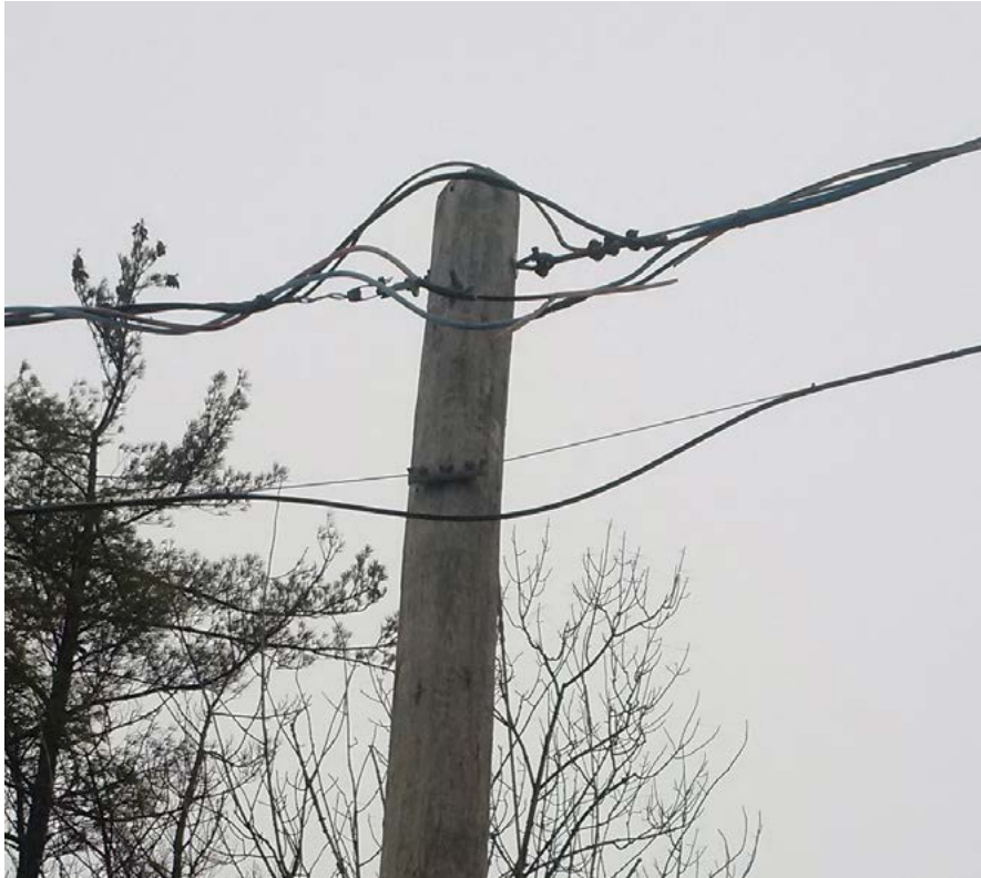
On aerial runs, be careful of how much slack is needed between poles.
